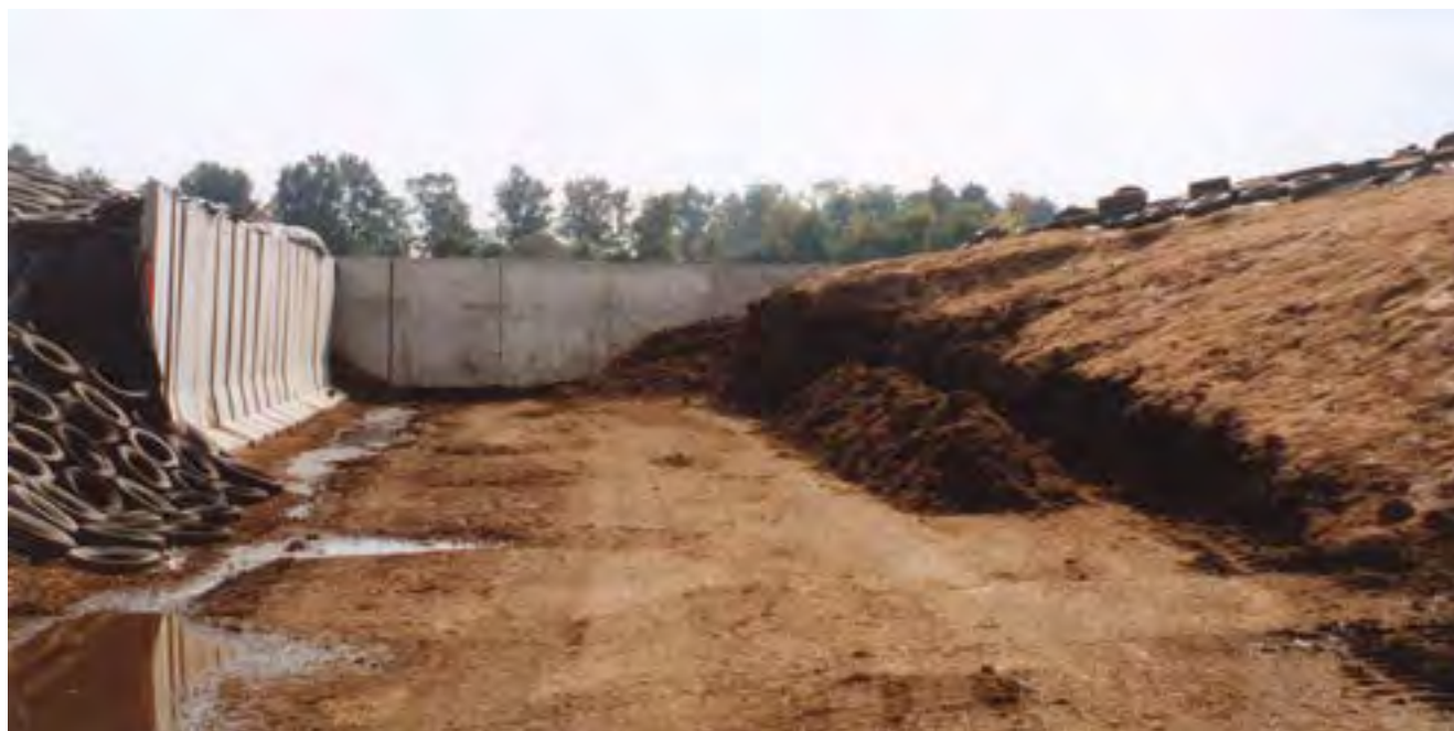
Figure 3.9.d. Bunker silos must be packed tightly to limit the amount of oxygen available to bacterial and plant fermentation. Driving of a packing tractor back and forth can lead to tractor rollovers. Credit: Penn State Extension Ag Safety Team
