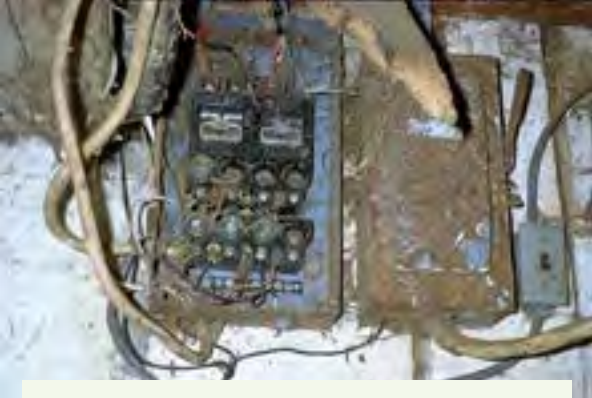
Figure 3.6.c. Improper electrical wiring methods and materials placed into a hostile farm environment can lead to fires and electrocution of people and livestock. Credit: Penn State Extension Ag Safety Team
