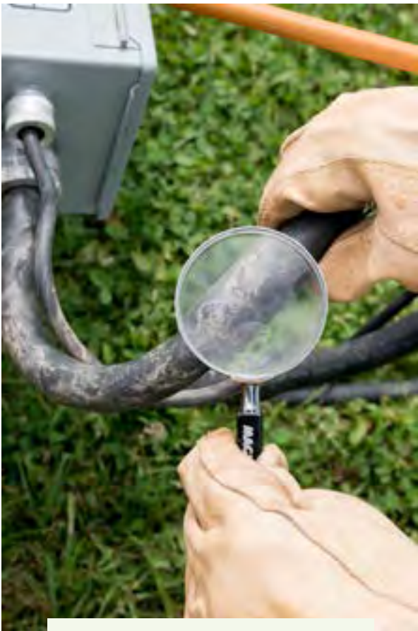
Figure 5.5.e. Use a mirror or piece of cardboard to check for high-pressure hydraulic leaks. Do not use your skin! Pinhole leaks are often invisible. Credit: Jeff Mathison
