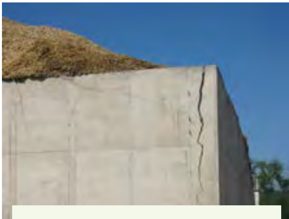
Figure 3.9.1.b. Bunker silo sidewalls are under great stress from silage weight and packing. A sidewall collapse could send a truck or tractor into an overturn. This situation must be repaired before harvest begins. Credit: Penn State Extension Ag Safety Team
