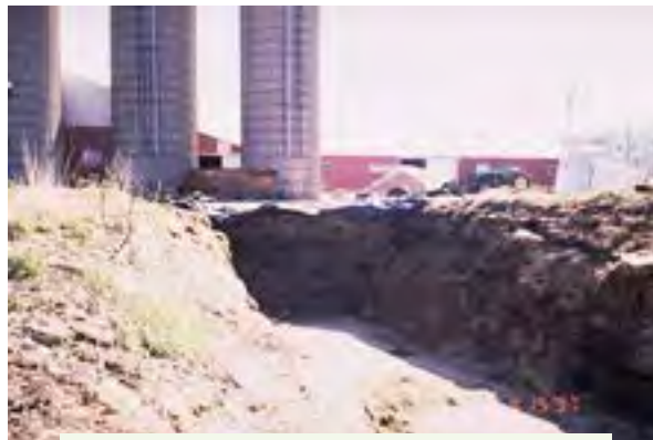
Figure 3.8.c. Trenches and pits in agriculture pose risk of sidewall cave-in and entrapment of the worker. Death by crushing can result. Suffocation can also occur. Credit: Penn State Extension Ag Safety Team
