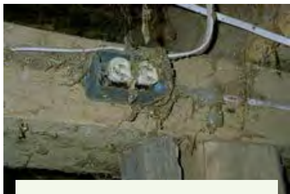
Figure 2.6.b. Barns and machine shops are dusty places. Unprotected electrical boxes can collect large amounts of dust and debris. This can start a fire by causing an arc across the conductors and igniting the debris. Practice good housekeeping and use electrical safeguards. Credit: Penn State Extension Ag Safety Team
