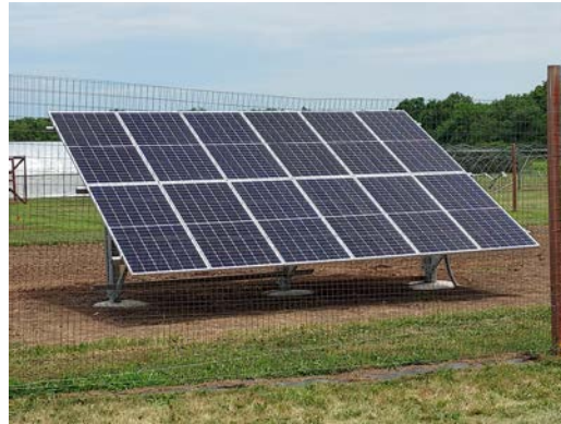
Solar array constructed over the summer provides renewable power for the irrigation and aerator pumps to water vegetable and turf research plots and keep the holding pond water circulating.
