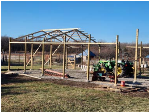
An outdoor classroom is being constructed just south of the Backyard Garden.
