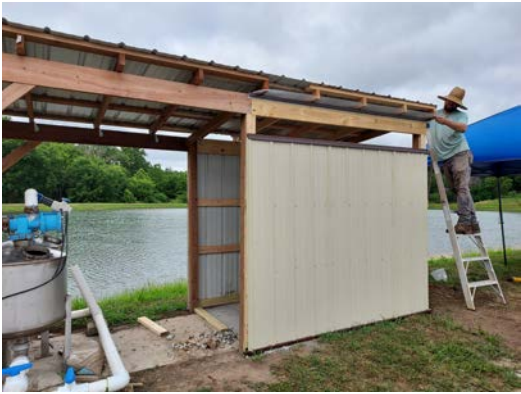
Solar Pumphouse nearing completion in July. The solar-powered pump will provide water for research plots by pumping from the holding pond. The pump also powers pond aerators.
